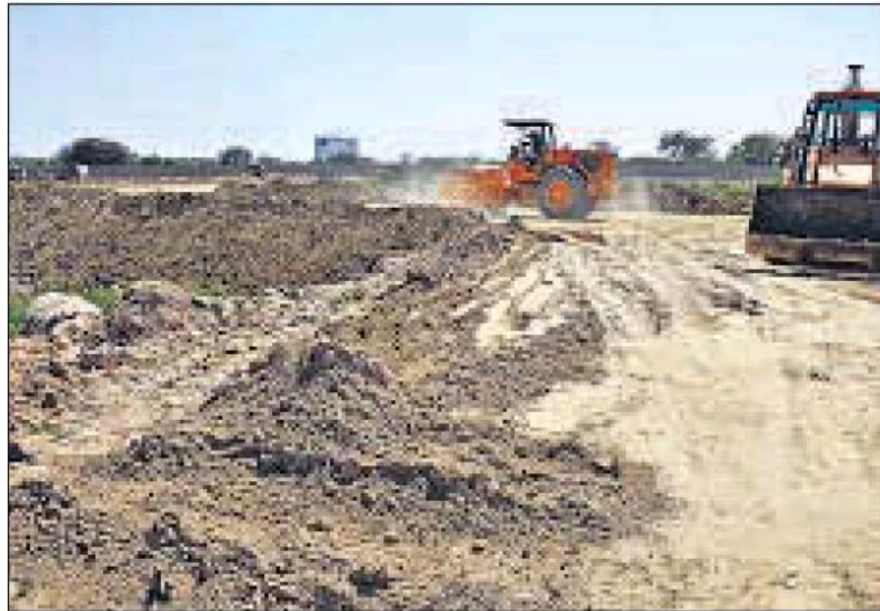
■ The shopping complex will come up here. A new Metro rail station will also come up at Botanical Garden.
